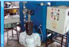
HIGH PRESSURE AND HIGH TEMPERATURE FACILITY
